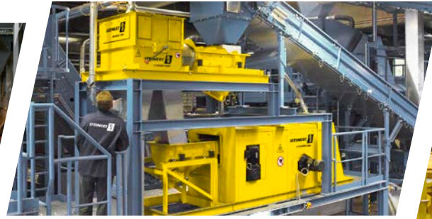
Removal of ferrous parts using STEINERT MOR
