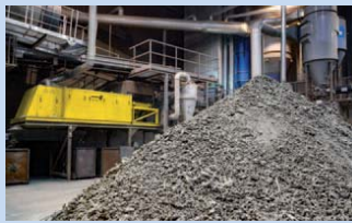
The non-ferrous metal separator recovers zorba up to 0.5 mm grain size from the IBA. Zorba is a mixture of non-ferrous metals such as aluminium, copper, zinc and brass.
